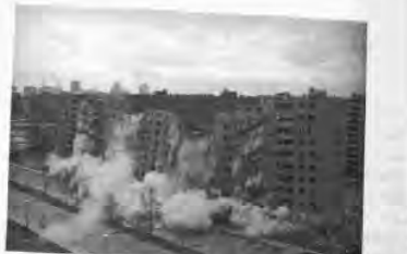
FIGURE 73 On April 21, 1972, the second 11-story building in the Pruitt-Igoe public housing complex was demolished by dynamite. © Bettmann/CORBIS.
