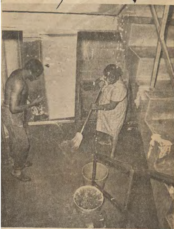
First-floor tenants at a Pruitt-Igoe apartment sweeping water that had run down the stairs from an upper floor where a fire hose fixture had been removed. (Post-Dispatch Photo)
